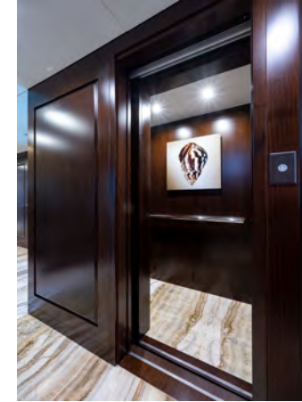
Elevator (Services all 4 Decks)
